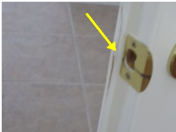
Master bathroom door - Crack in trim.
