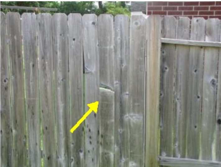
Fence board needs repair
