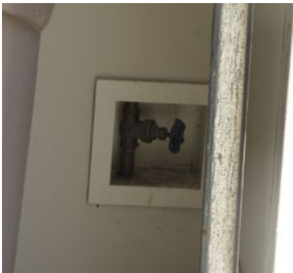
Main water shutoff.
