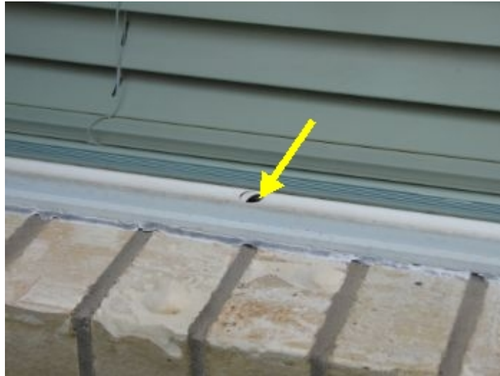
Small chip missing from North window trim.
