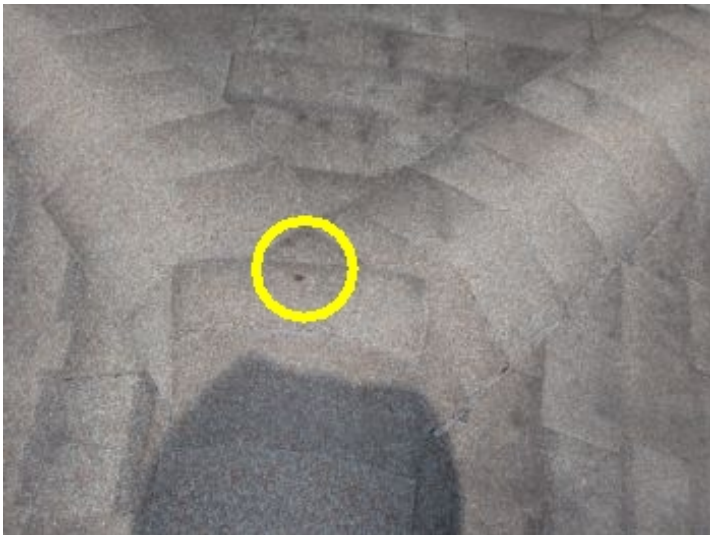
Nail need to have sealant applied.
