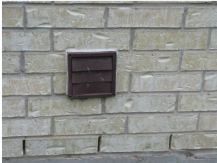
Dryer vent located on South wall.
