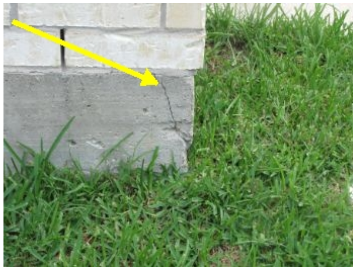
Small settling crack in foundation. SE corner.
