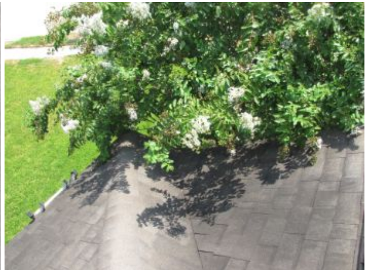
Trees need to be trimmed away from roof.
