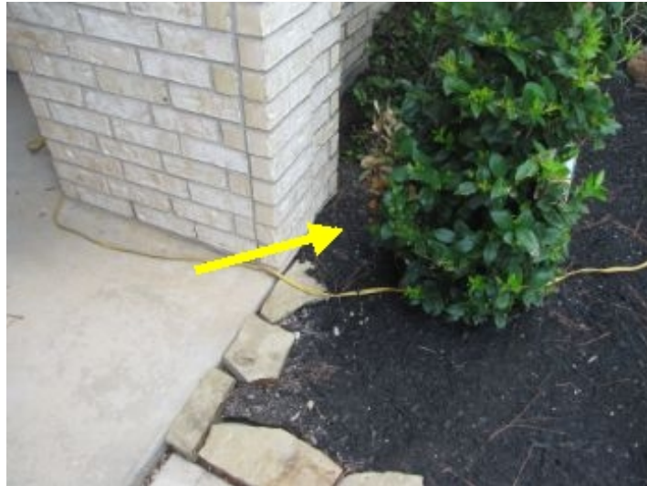
Topsoil in beds too high - should have 4" from bottom of first row of bricks.
