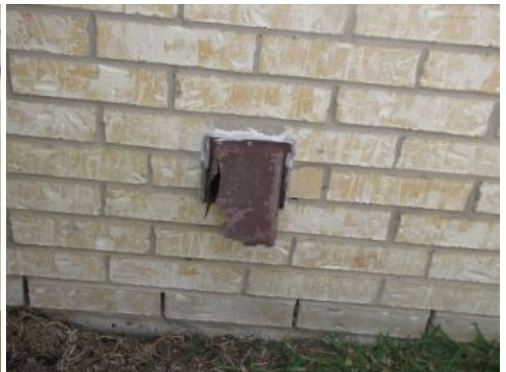
Air vent for fireplace needs repair.
