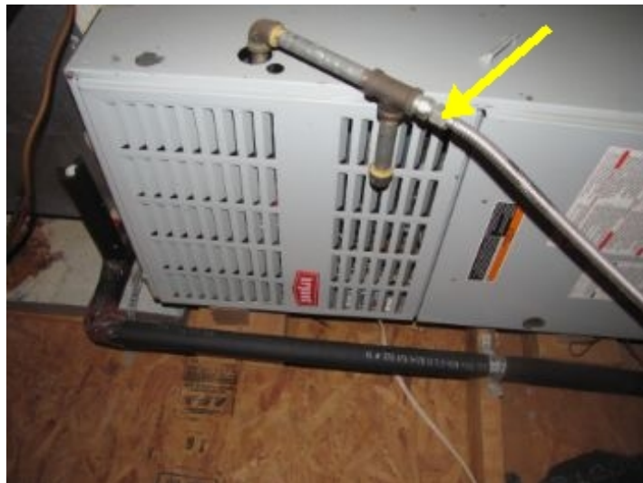
Furnace gas line checked for leaks - None detected.
