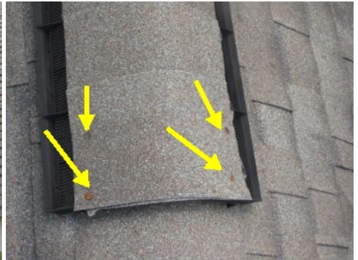
Nails need to have sealant applied - Ridge Vent
