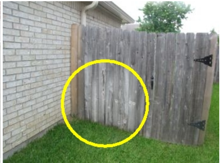
North side fence pickets showing wear
