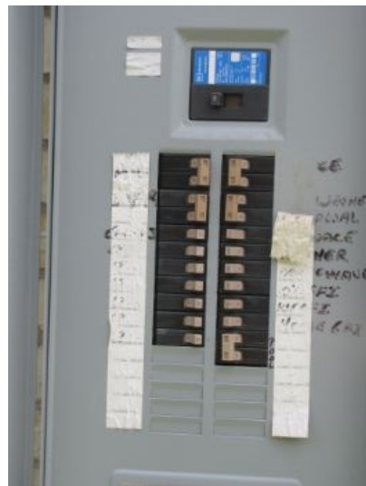
Electrical box labeling difficult to read.
