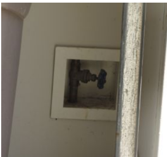
Main water shutoff.
