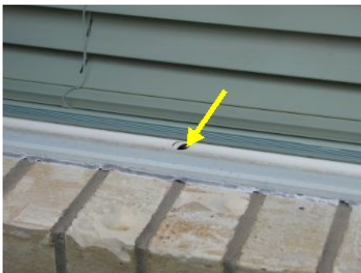
Small chip missing from North window trim.
