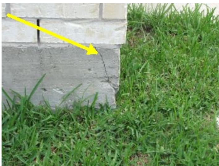
Small settling crack in foundation. SE corner.
