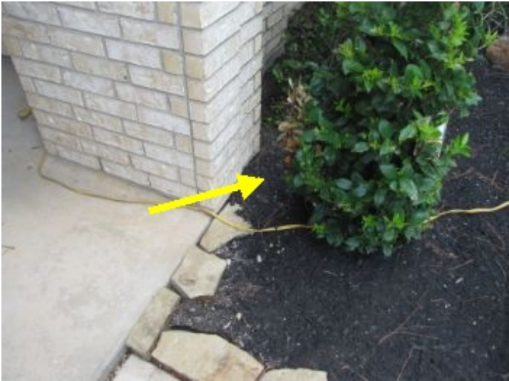
Topsoil in beds to high - should have 4" from bottom of first row of bricks.
