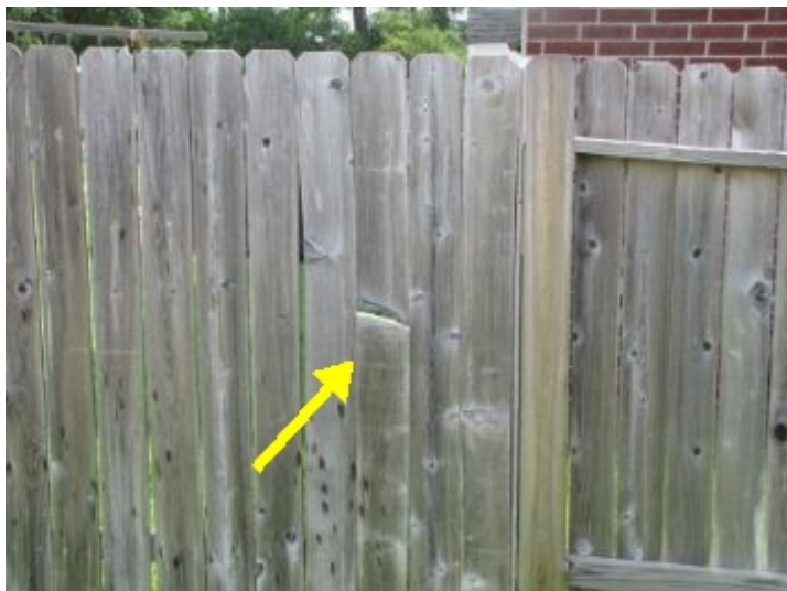
Fence board needs repair
