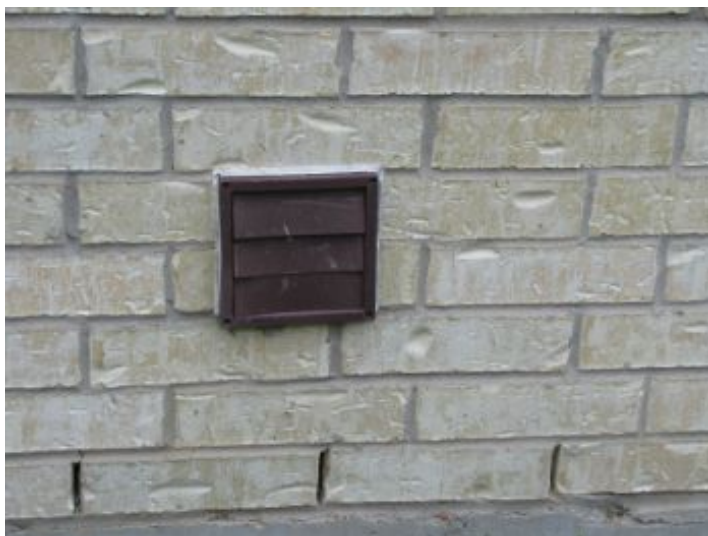
Dryer vent located on South wall.
