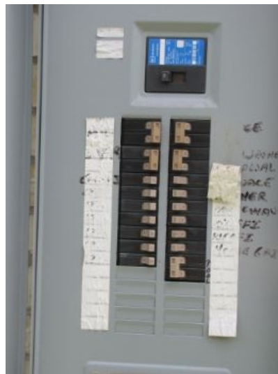
Electrical box labeling difficult to read.
