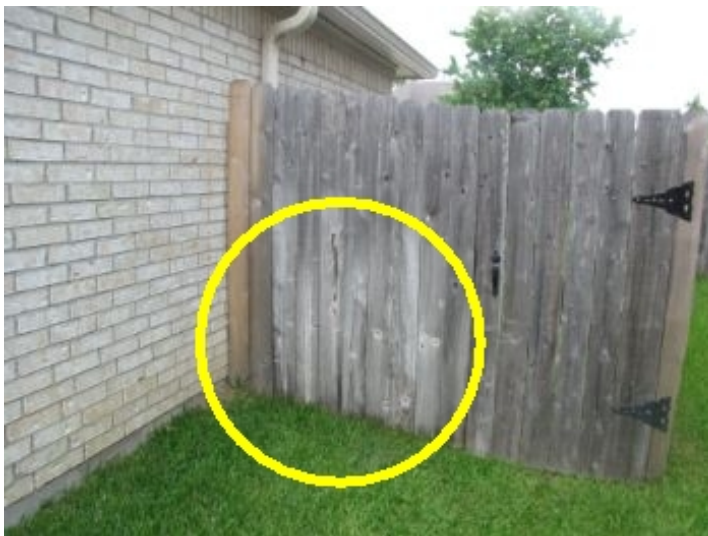
North side fence pickets showing wear
